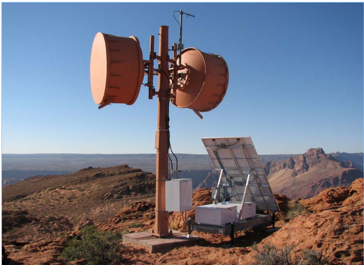
Figure 6 RF Repeater Installation with Solar Power
